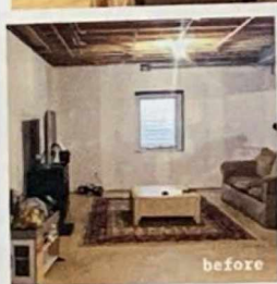
BEFORE Unpainted drywall lined an ad hoc TV area for the kids. Pipes and conduit loomed overhead in the open ceiling.
